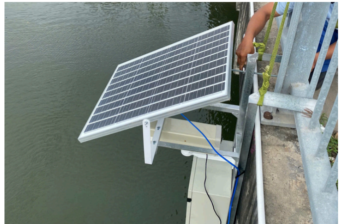
AI-CCTV at Can Tho, Vietnam
